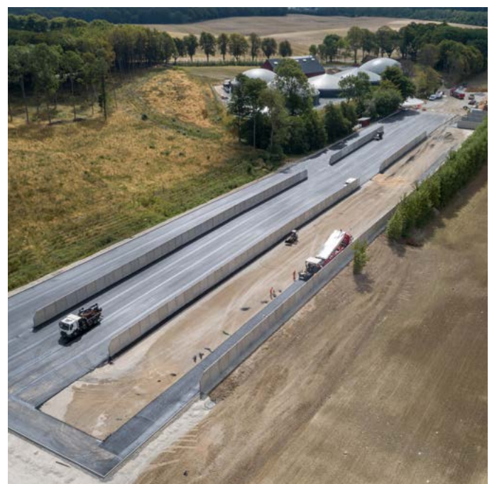
Colas laid asphalt in Frijsenborg Biogas' 11,000-square-metre trench silo in just two days in July 2018.
